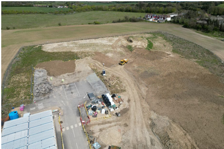
Image above shows demobilisation of old site offices in Section 2 and reinstatement of the area.
