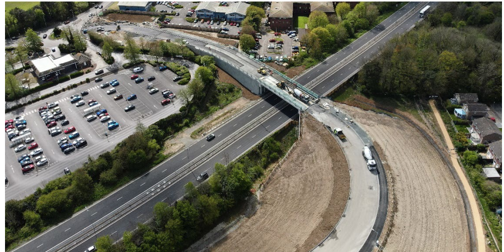
Image above shows Sections 1B North (new bridge and embankment) and 1B South (towards Tesco roundabout) and construction of asphalt.
