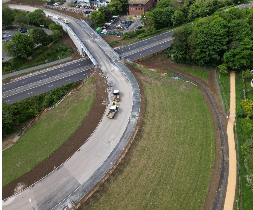
Image above shows Sections 1B North (new bridge and embankment) and 1B South (towards Tesco roundabout) and construction of asphalt.
