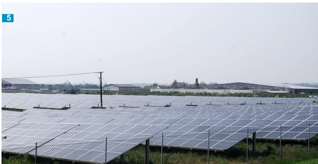
5. Solar arrays near Richborough
